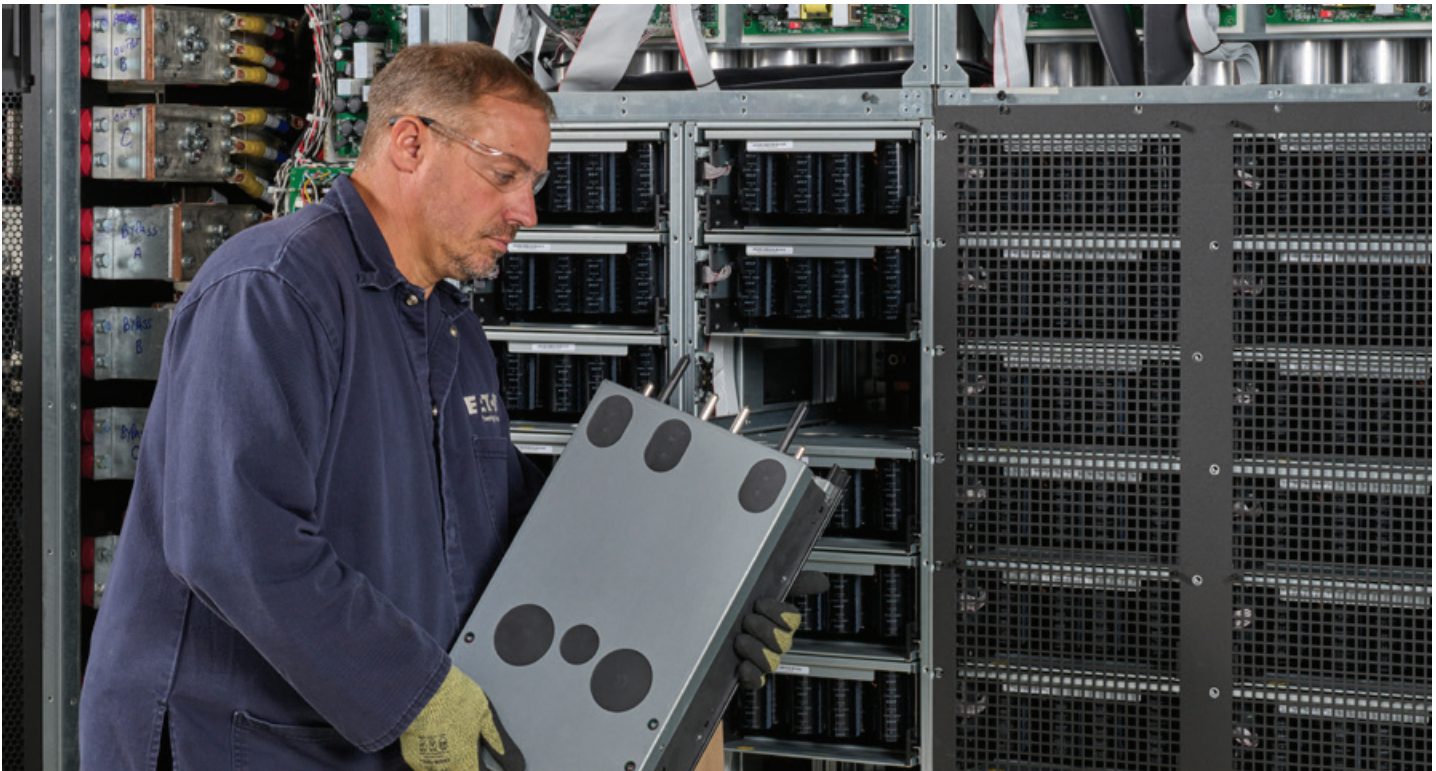
Eaton technician inspecting an Eaton 9395XC UPS.
