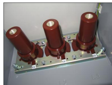
Cones type C Load-break switch 630 A without current transformers
