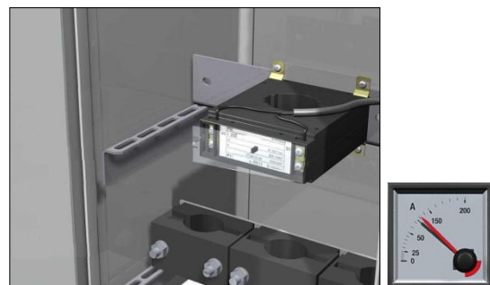
Current transformer and ammeter
