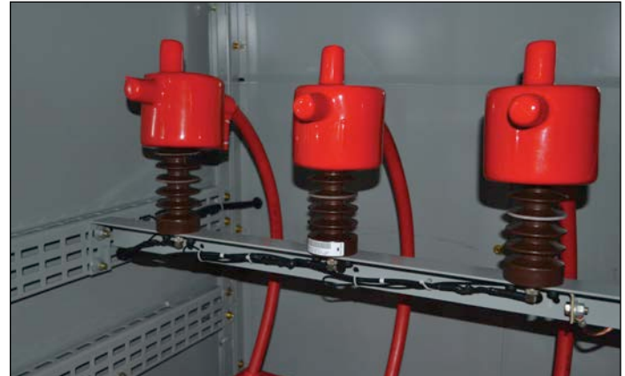
Figure 5.4-5. OVS Sensors Mounted in Cable Compartment
