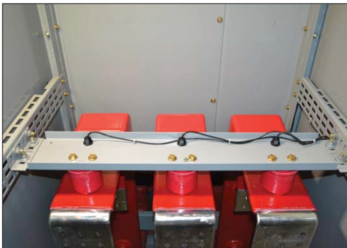
Figure 5.4-7. Typical Install for Continuous Thermal Monitoring Sensors
