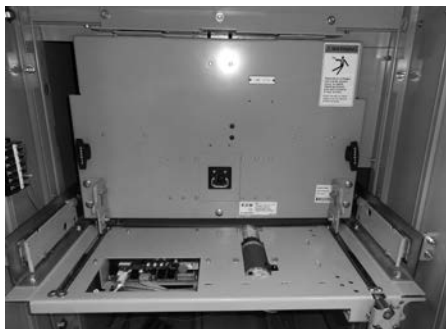
Type VC-W Standard Switchgear Auxiliary Drawer with Type MR2 Integral Racking
