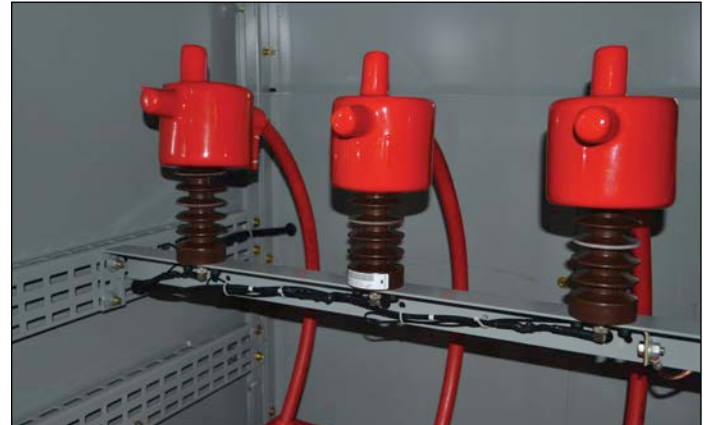
Figure 5.1-8. OVS Sensors Mounted in Cable Compartment
