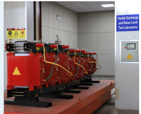
Partial discharge laboratory
